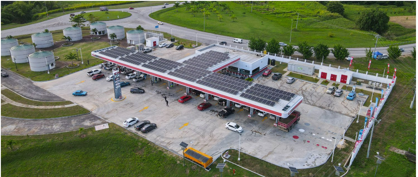
FIGURE 1: 320 SOUTH FACING SOLAR PANELS AT THE PREYSAL SERVICE STATION WHICH FORM PART OF THE PV SYSTEM.
